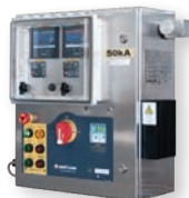
WATCONNECT™ control panel
